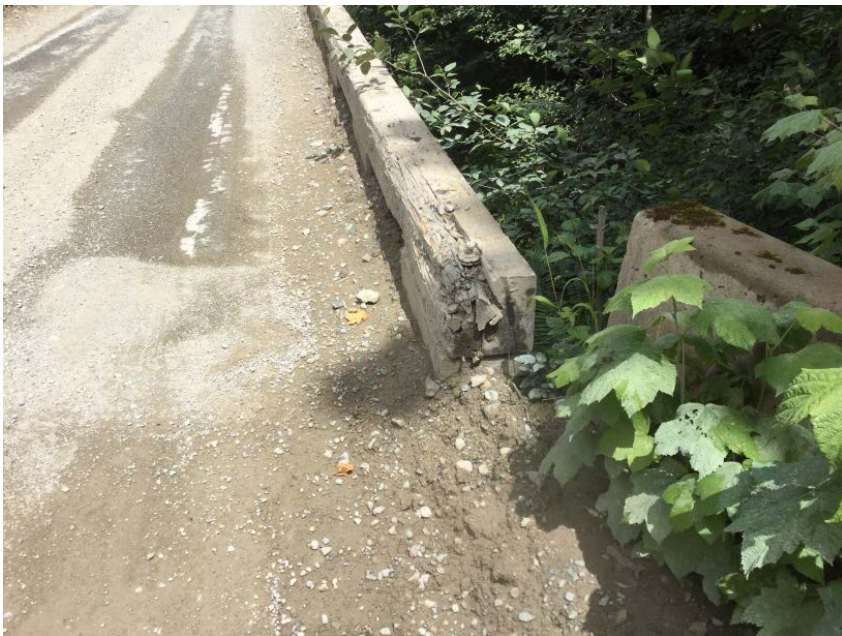
Damage noted to right approach rails
